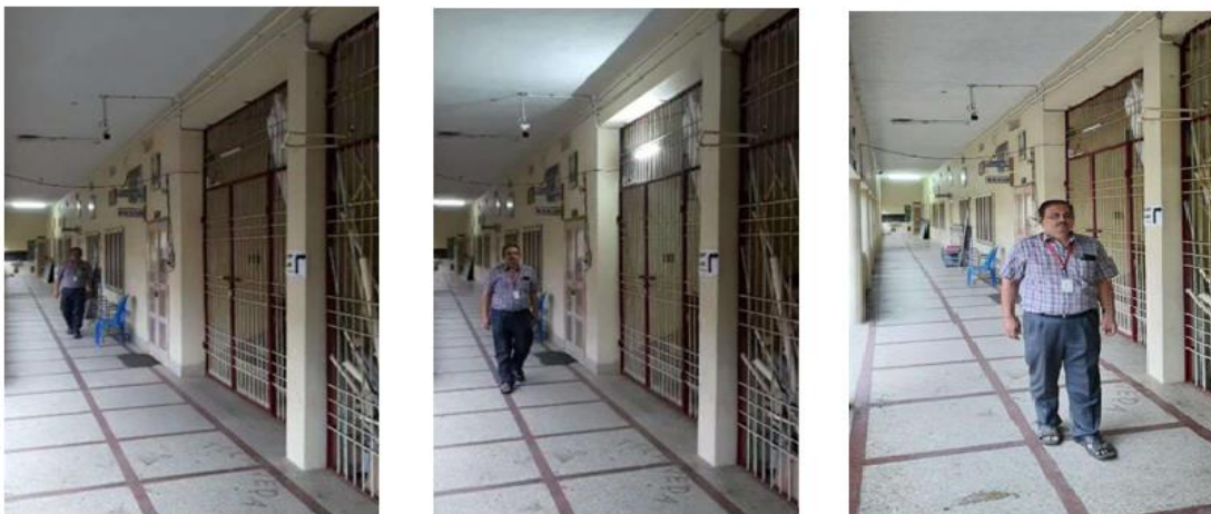
Figure - PIR BASED LED LIGHT AT THE ENTRANCE OF THE BLOCK
